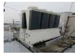
High-efficiency refrigerating machine [Kakogawa-higashi Plant]
