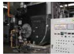
High-efficiency steam boiler (FT boiler) [Kakogawa-higashi Plant]
