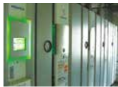
High-efficiency steam boiler [Takasago Plant]
